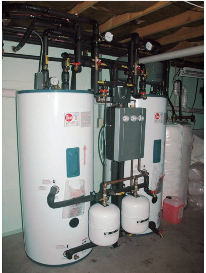
The balance of system components of the solar hot water system.
