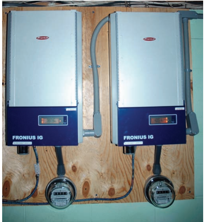
Two Fronius grid-tied inverters make up the balance of the home's photovoltaic system.
